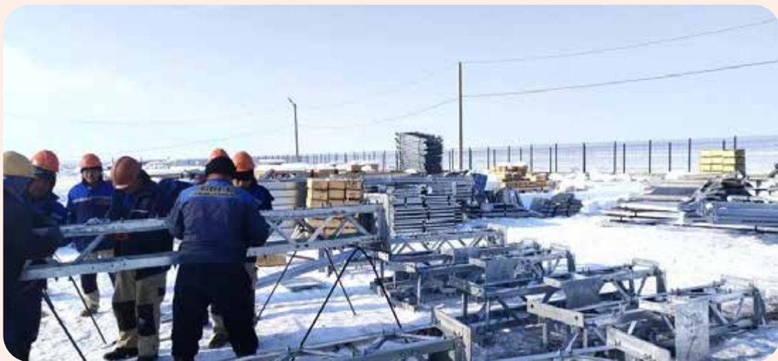
The Zafarabad 220 kV Substation Project
