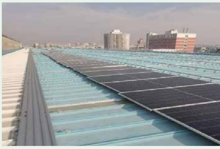
Shanghai Electric Turbine Plant Rooftop PV
