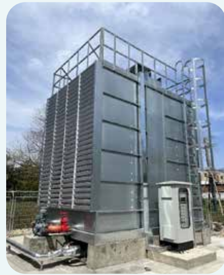
Green hydrogen production-storage-use integrated demonstration project of Shanghai Electric
