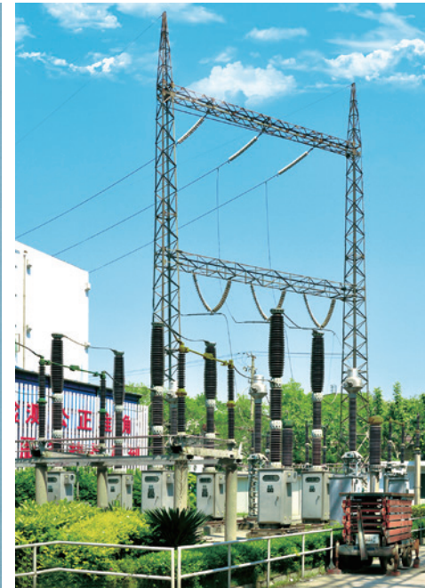
220kV 户外开关站 220kV Outdoor Switching Station
