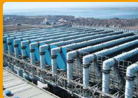
Mechanical Draft Air Cooled Condenser (ACC A-Frame)
