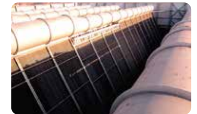
Shanxi Zhongyu Bundles Rebundling 2x135MW
